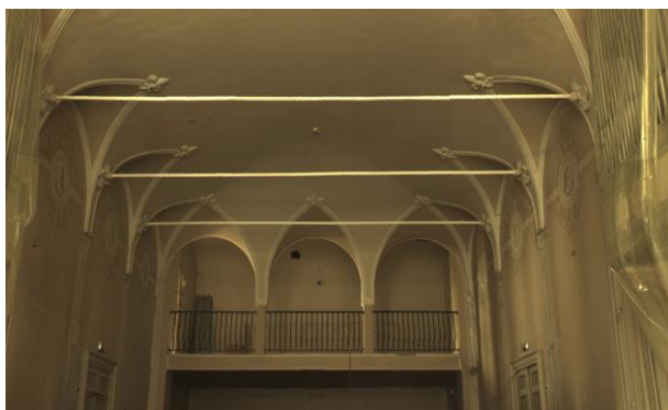
Figure 2. The nailed and lowered profile pavilion vault which covers the Sala Verdi of Conservatorium, in Parma (Italy)
