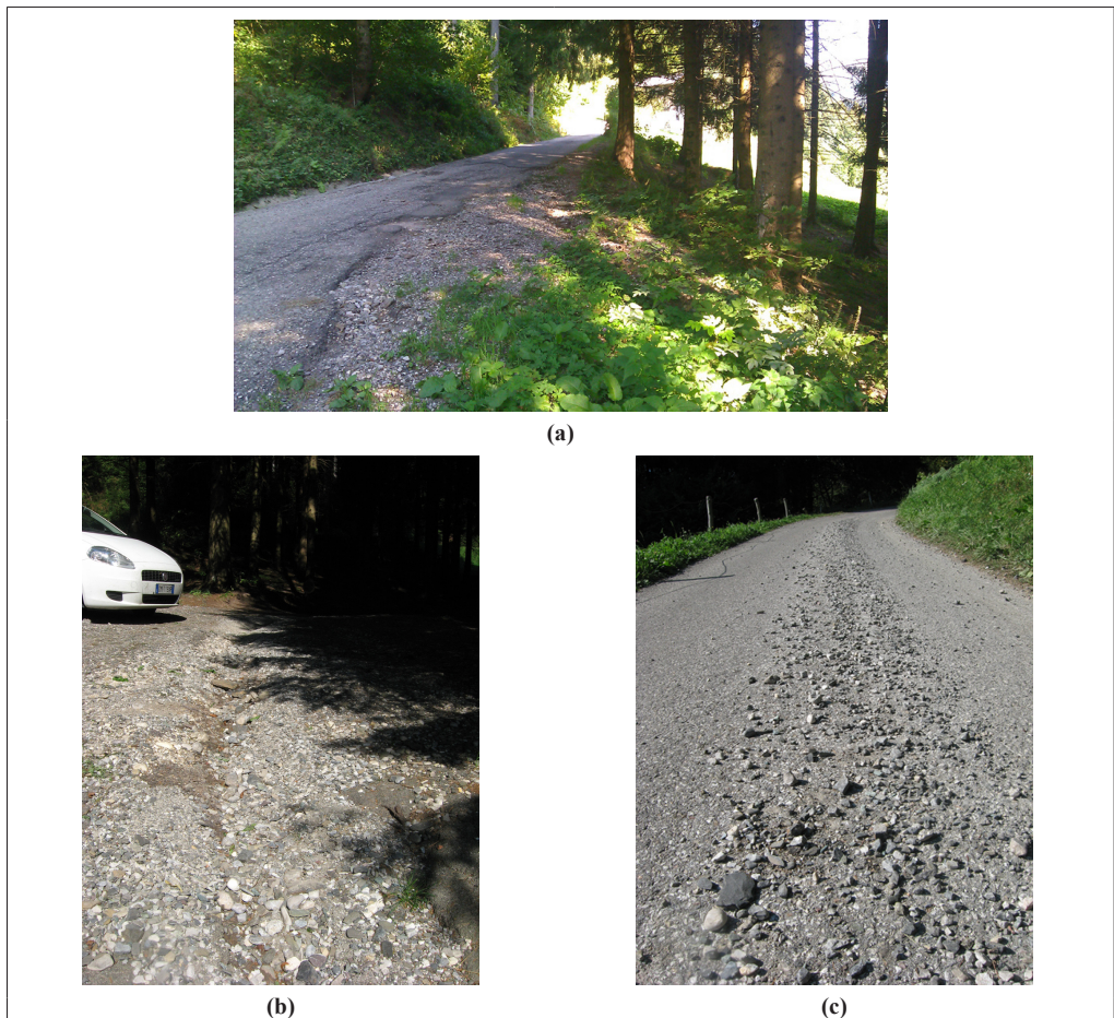
Figure 4 - Case study P2 of Paularo showing: (a) the road section subject to flow direction alteration, (b) erosion outside the road, and (c) sediment deposition along the road.
