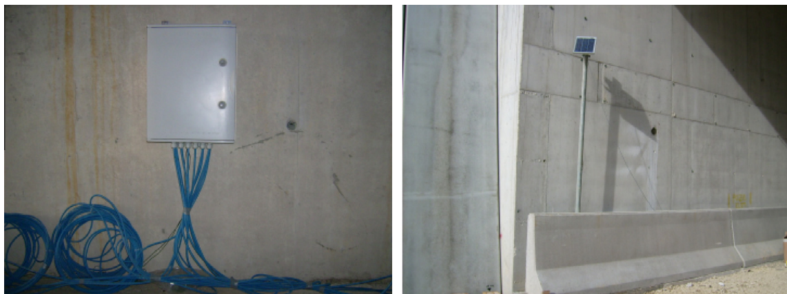
Fig. 5. Wall-mounted data logger powered by the solar panel placed outside the tunnel.
