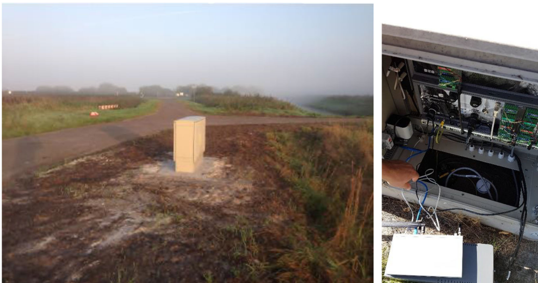
Fig. 6 Exterior (left) and interior (right) of a G-station. The stations were installed in remote locations to minimize the noise recorded
