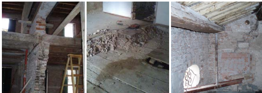
Fig. 2 Building envelope before renovation: a) crooked walls; b) demolished partition walls left and used as a substrate; c) beam support in the perimeter wall.
