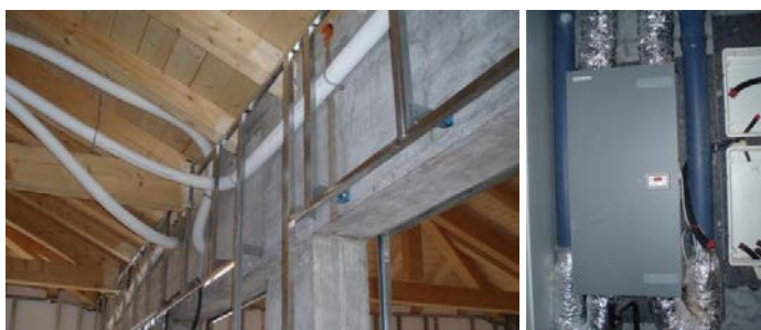
Fig. 5 Mechanical ventilation system.
