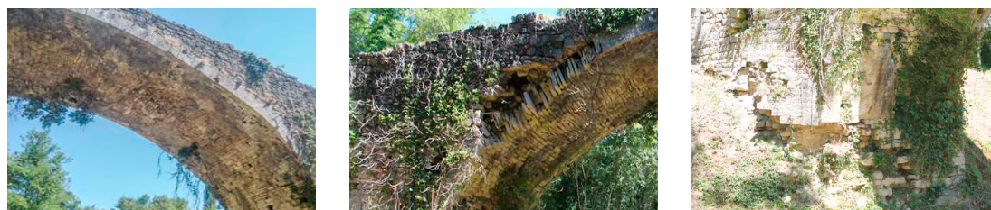
Fig. 2. Structural details: (a) cracks on the vault, (b) material detachment from the voussoir and (c) damage of the West abutment.
