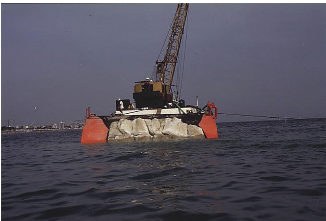
Fig. 6. Construction techniques: the geotextile and the whole cross section, sliding over a suitable slipway, are laid down from the pontoon.
