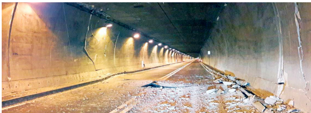
Fig. 1 - Details of the damaged road surface in the San Benedetto tunnel (after Galli et al., 2017)
