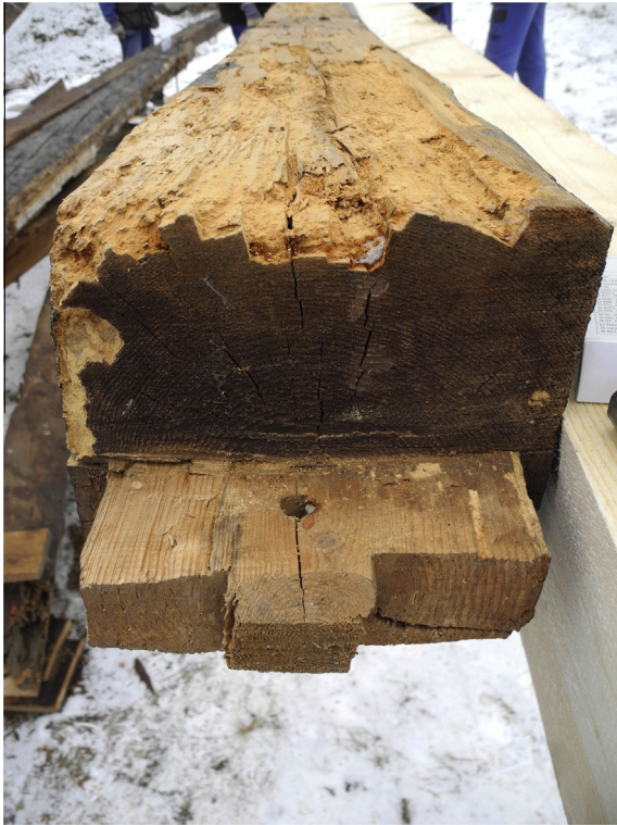
Fig. 27. A detail of damage to a tie beam, which was left in the original position.
