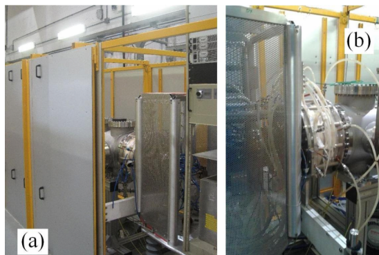
FIG. 2. (a) View of the NIO shielding box with main door open and main rf generator removed; (b) accelerator column and HVD view from the opposite side.
