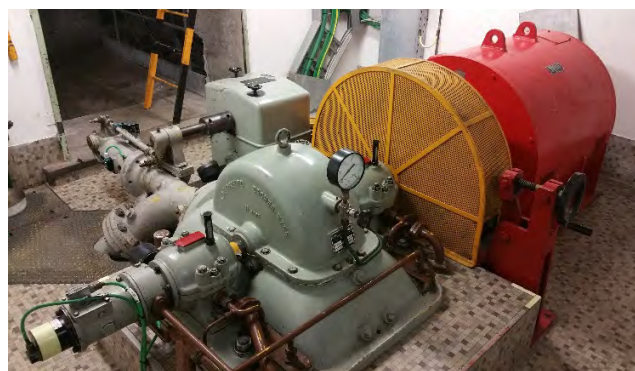
FIGURE 4. Emergency generating set reserved for hydro power plant auxiliary systems.
