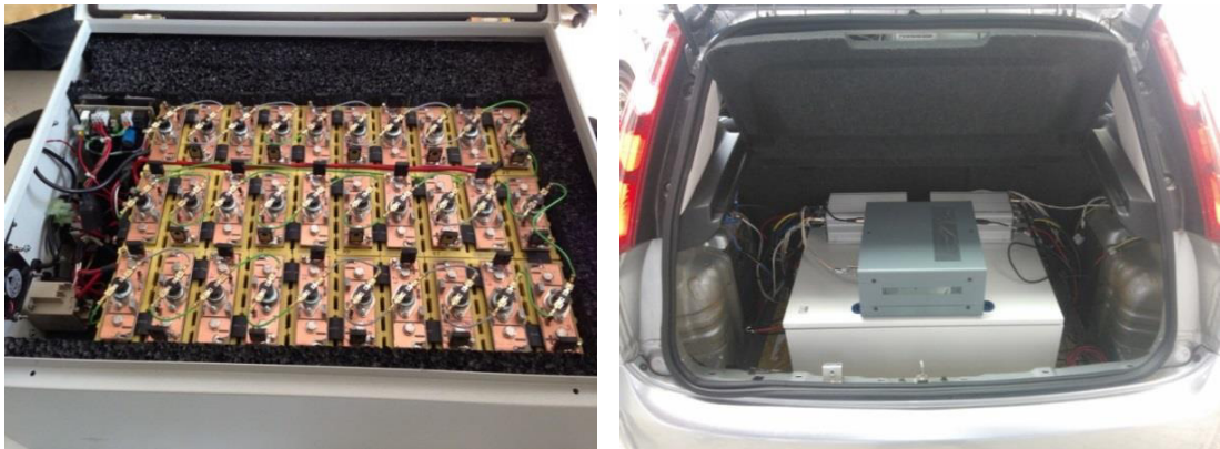
Fig. 6. Lithium-Ion battery pack installed in the FIAT Grande Punto.
