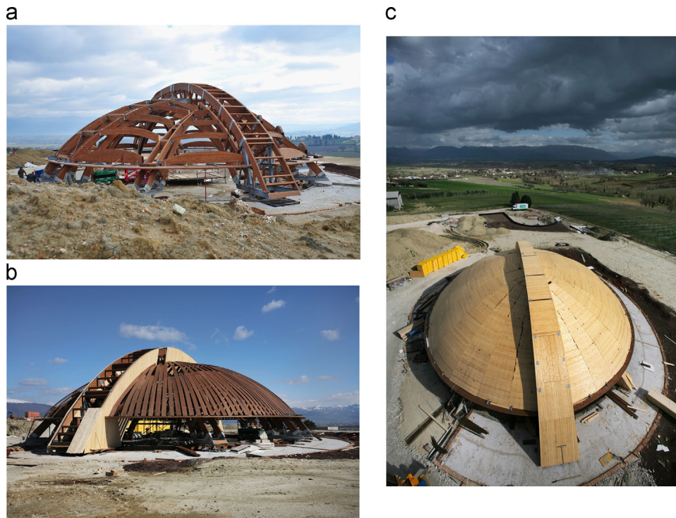
Figure 5 Steps in constructing the Carapace structure on which the wood ribs are visible.
