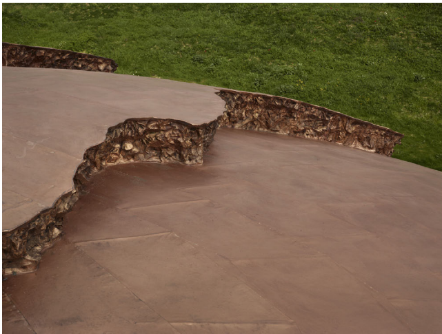
Figure 10 Detail of a cut on the roof.
