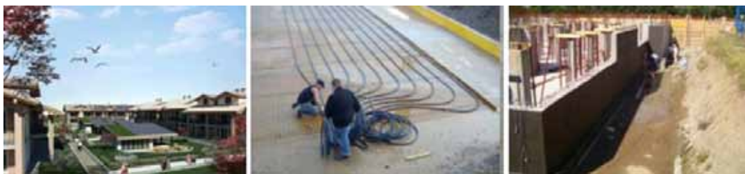
Fig. 1. (a) render view of the complex; (b, c) views of the construction site.
