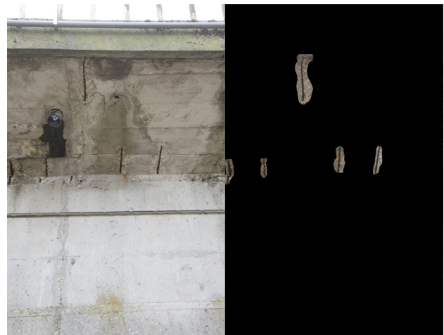
Figure 6. Detailed image of the slab intrados, at right recognized damages
