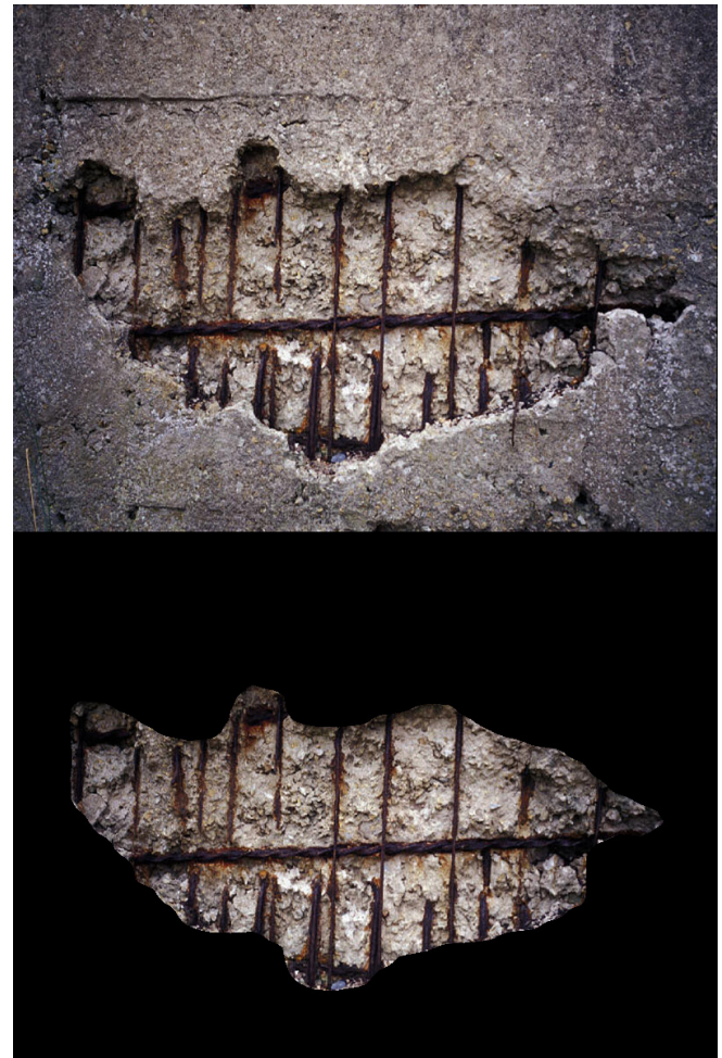
Figure 3. Example of spalling detection
