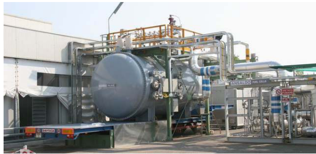
Figure 2: Ansaldo MCFC plant at Bosco Marengo site.
