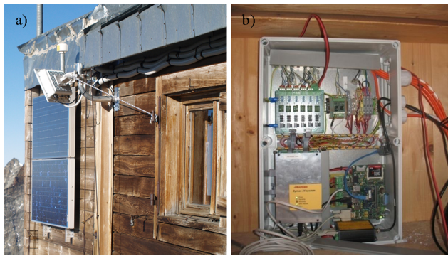
Fig. 3. (a) The solar panels, the GPS and the aerial radio installed outside the Carrel hut; (b) the acquisition system installed inside the hut (photo by Signori and Bani, 2010).
