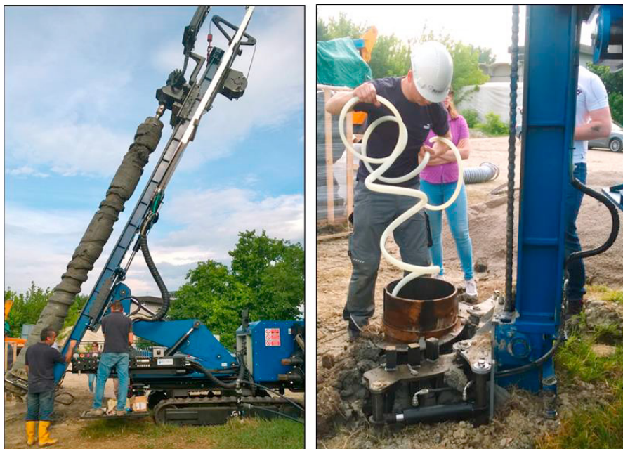
Fig. 2. Some installation phases of the newly developed Helix GSHP at the Molinella test site.
