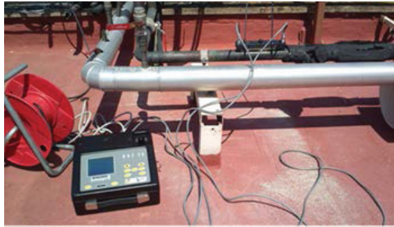
Fig. 12. primary flow measurement with a portable ultrasonic flowmeter
