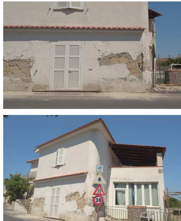
Figure 10. Images of damages by UAV of a building in Lacco Ameno
