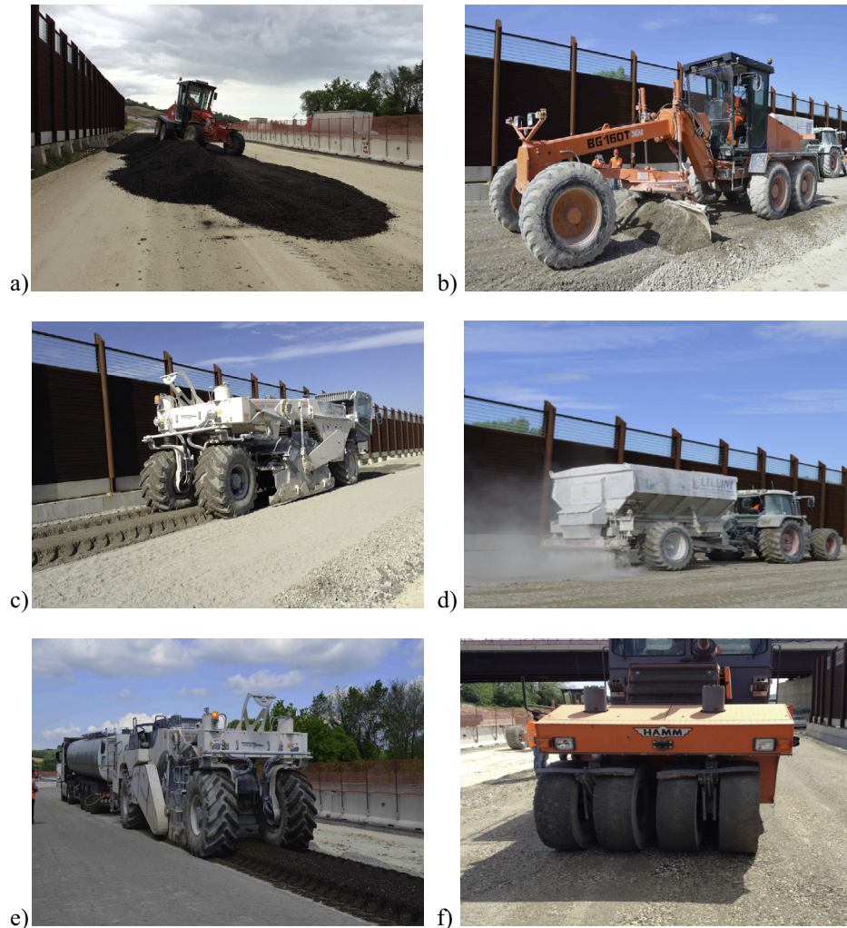
Fig. 3. Construction of CBTM and CTM layers: (a) RAP material restoring; (b) placing of RA g layer; (c) mixing of the milled material; (d) spreading of cement; (e) stabilization with bitumen emulsion; (f) final compaction.
