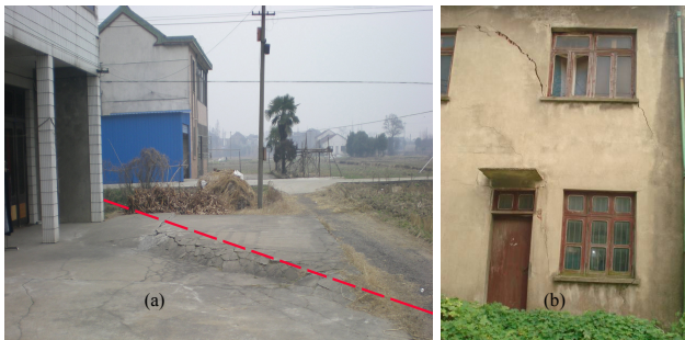
Figure 2. The ground rupture (a) and damaged house (b) at Guangming Village (red line in (a) shows the direction of the earth fissure).
