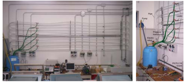
Fig.4. System mounted on the wall.
