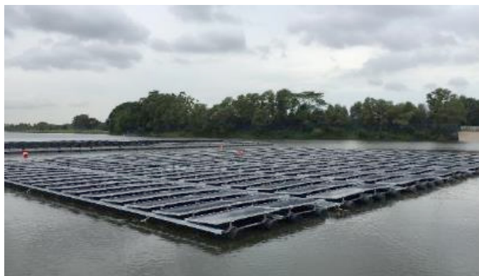
Figure 10. Floating photovoltaic system (rating 100 kWp) in Tiengheh reservoir in Singapore
