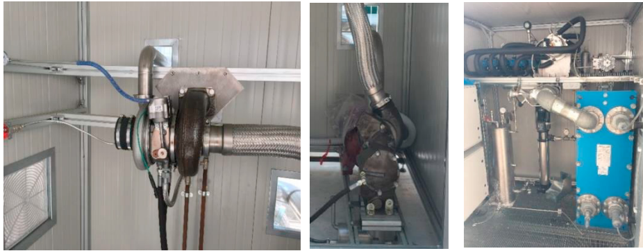
Fig. 3. Turbocharger (left), power turbine (center), steam turbine (right)
