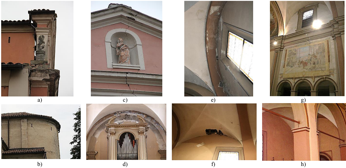
Figure 2. Observed damages after the Emilia Romagna Earthquake. a, b) Overturning of the structural elements. c) Overturning of the tympanum. d, e, f) Detachment of the vaults from the walls. g) Diagonal cracks in the chorus walls and h) longitudinal tie rods.
