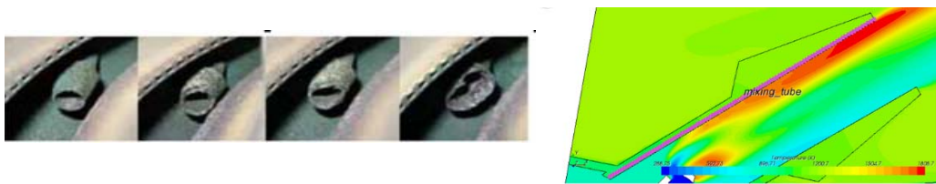
Fig. 2. High temperature corrosion of mixing tube [26] and its CFD explanation by the authors [21, 25]
