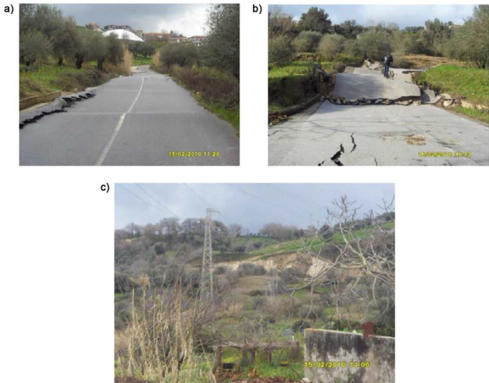
Fig.2. (a,b)cracks and bulges along the SP 55 road; (c)increase in the height of a pre-existing scarp at 270 m a.s.l.(location is indicated in Fig.1).
