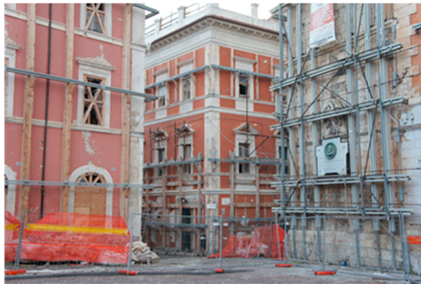
Fig. 2. Palazzo Bruni-Riga after the earthquake: angled facade on Via Cavour and Via delle Aquile. On the right the basement of bell tower.
