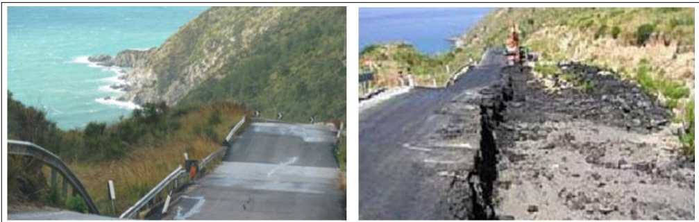
Figure 4 - Roadway deformation and deep cracks in the road.
