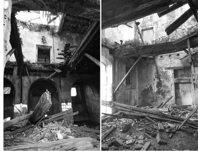
Figure 7. Internal collapses denounce the state of abandonment and the impossibility of detecting some Casale's areas.
