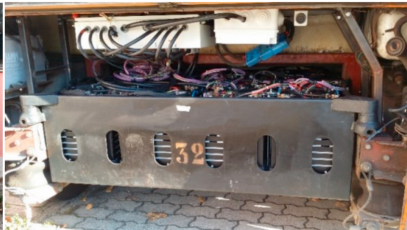
Figure 3 New battery pack installed
