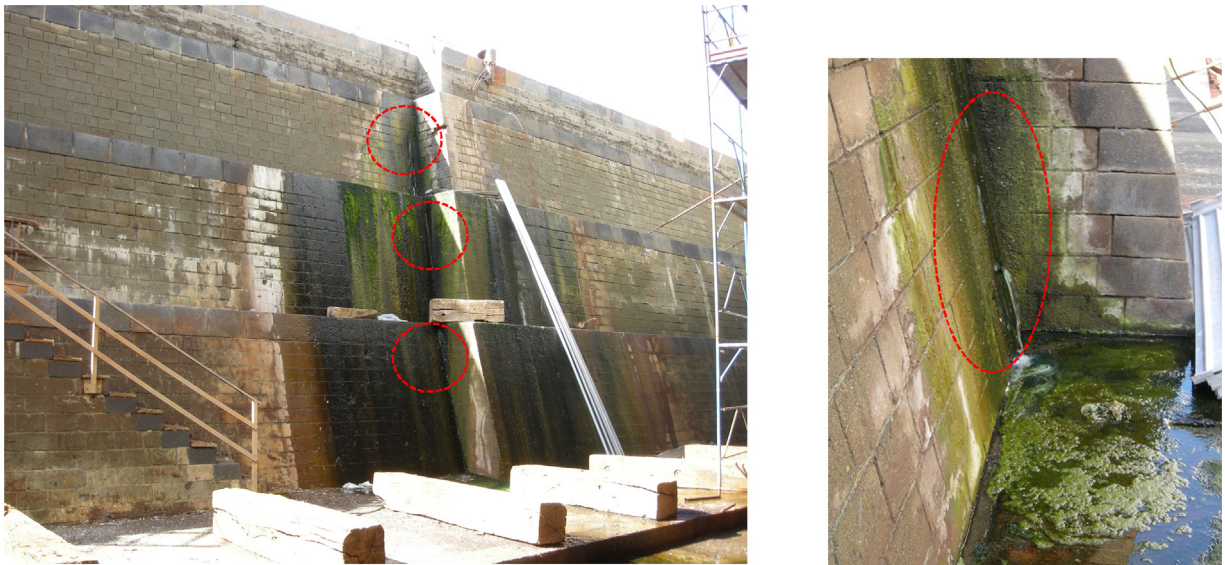
Fig. 26. Existing cracks in walls of Section CC (the most evident in red).
