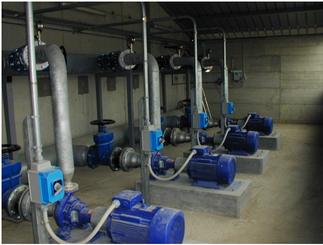
Figure 1. Casale pumping station: the four pumps in parallel.
