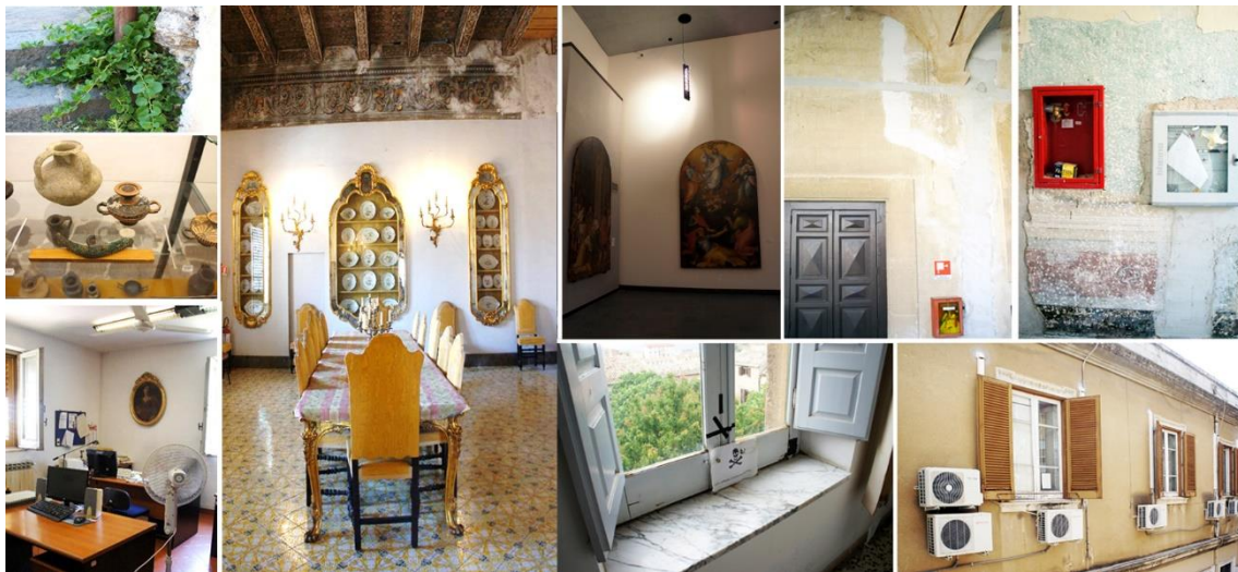
Figure 2. Collection of examples: buildings and artworks with poor maintenance conditions; implants insertion without an explicit logic. (Photos by Buda 2018)
