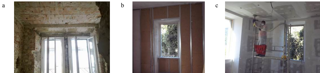
Fig. 4. Progress of the retrofit intervention: (a) wall and ceiling without plaster; (b) hemp fiber panels mounted on steel frames; (c) cellulose flocks blowing on the ceiling.
