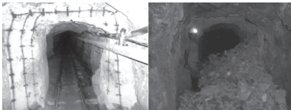
Figure 5 Preparation and result of the demolition blast of the concrete wall. In b/w for a better resolution of the pictures taken underground. In b/w for a better resolution of the pictures taken underground
