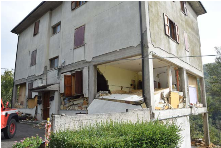
Fig. 1. Collapse of infills in a negligibly damaged rc frame (Pescala del Tronto, Italy, 2016).
