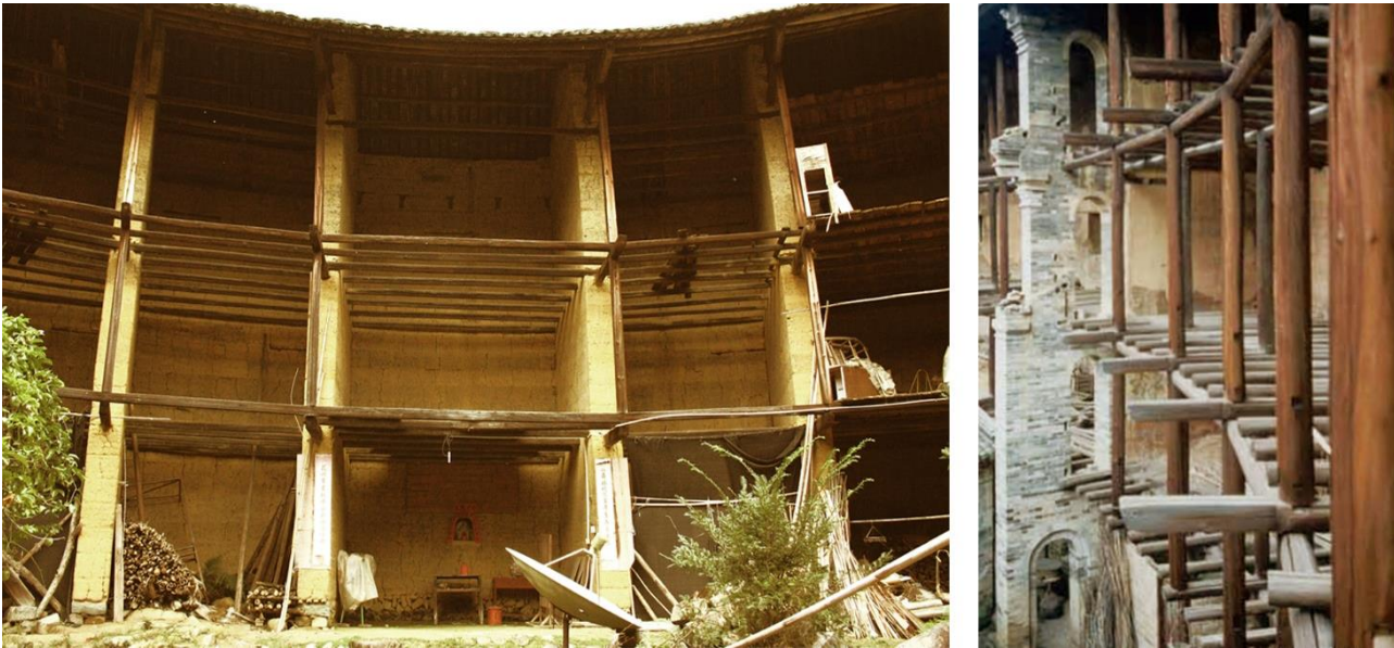
Figure 3. On the left, a Minnan Tulou with rammed earth load-bearing walls and wooden beams; on the right, a Hakka Tulou with wooden frameworks (2018, picture taken by E. Colafranceschi).
