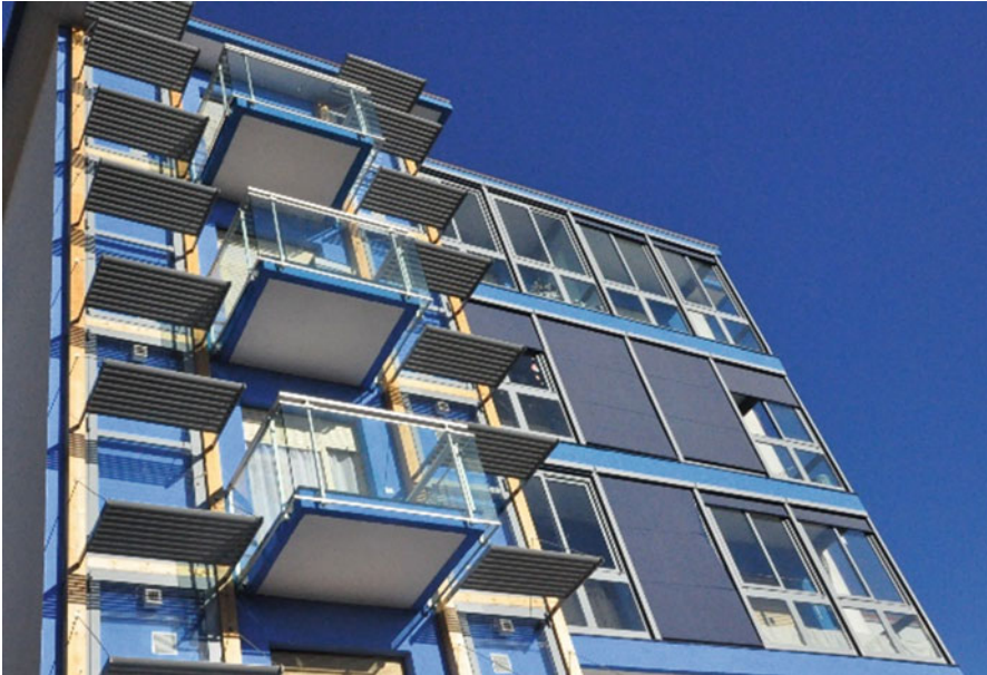
Fig. 57.1 Building B, one of the monitored buildings, after retrofitting: left : Trombe–Michel walls; right : solar glasshouses
