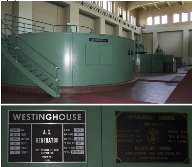
Figure 7. Saryyar Hydroelectric Plant, turbines
