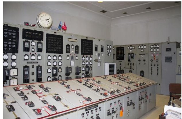
Figure 6. Saryiar Hydroelectric Plant, control room
