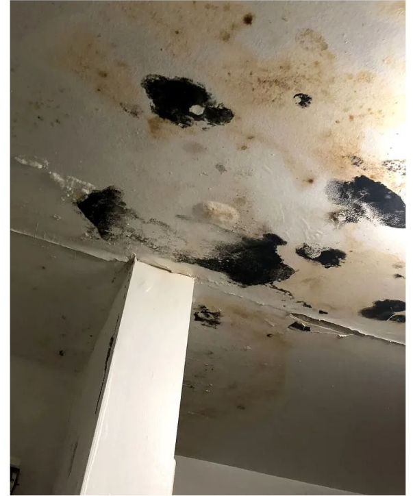
— Mold on the ceiling of an apartment in the Clay Arsenal complex in Hartford, Connecticut, which was owned by Emmanuel Ku. The Rev. AJ Johnson
