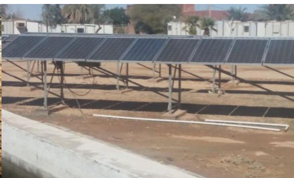
Figure 3. PV System at URERMS – ADRAR-Algeria
