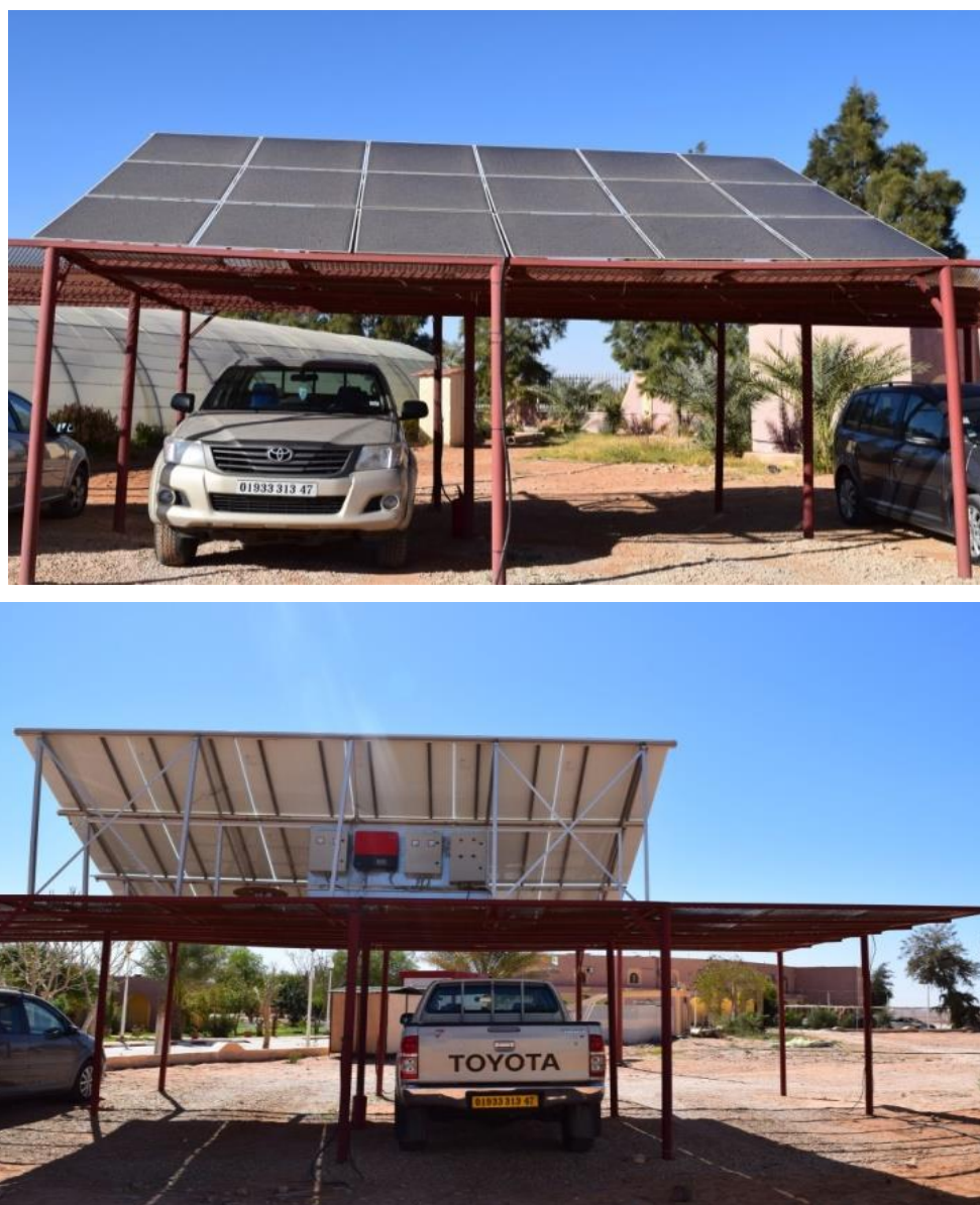
Fig 1. A PV station installed in Applied research unit Ghardaia
