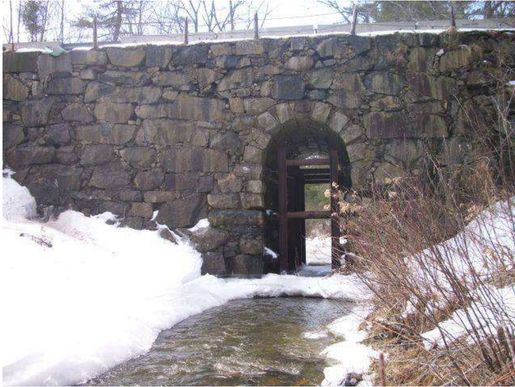
Figure 11. Steel structure in the arch of Stackpole Bridge prior to rehabilitation (Maine Preservation)
