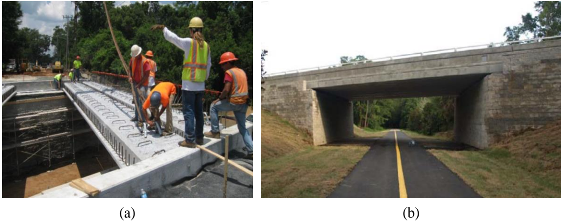
Figure 2.23: (a) Placement of FSBs adjacent to each other and (b) finished pilot project SRS 373 [51]
