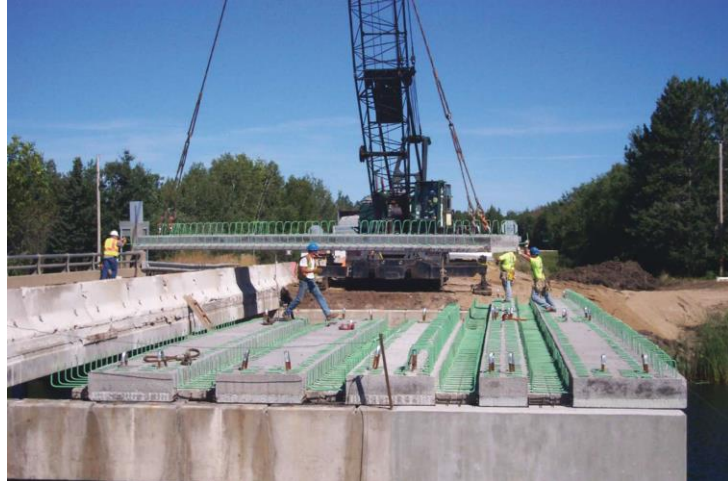
Figure 2.16: Erection of Bridge 04002 located on MN Highway 72 over the Tamarac River near the rural, northern Minnesota town of Waskish. [47]
