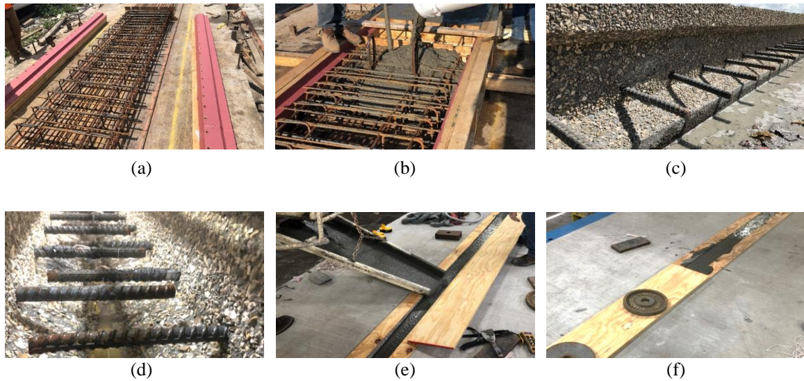
Figure 6.3: Slab beam and joint construction process: (a) reinforcement cage and wood formwork with painted paste retarder, (b) concrete cast in beams, (c) exposed aggregate finish, (d) joint geometry with non-contact lap spliced rebar, baker rod and leakage sealer, (e) wooden strips for UHPC overpour, and (f) top joint form closure application
