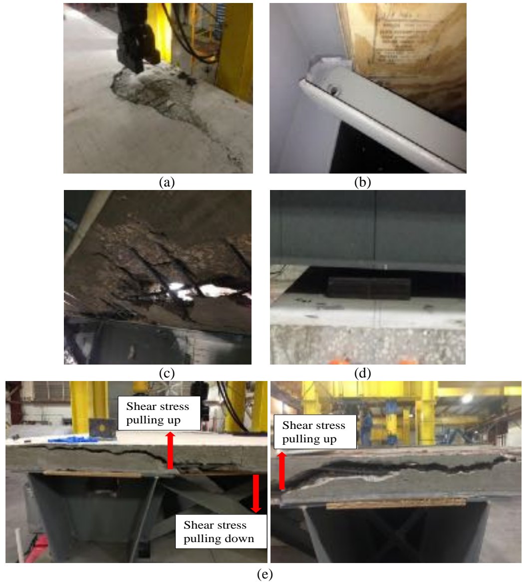
Figure 2-37. Damages in the Test E-1 of FIU bridge.
