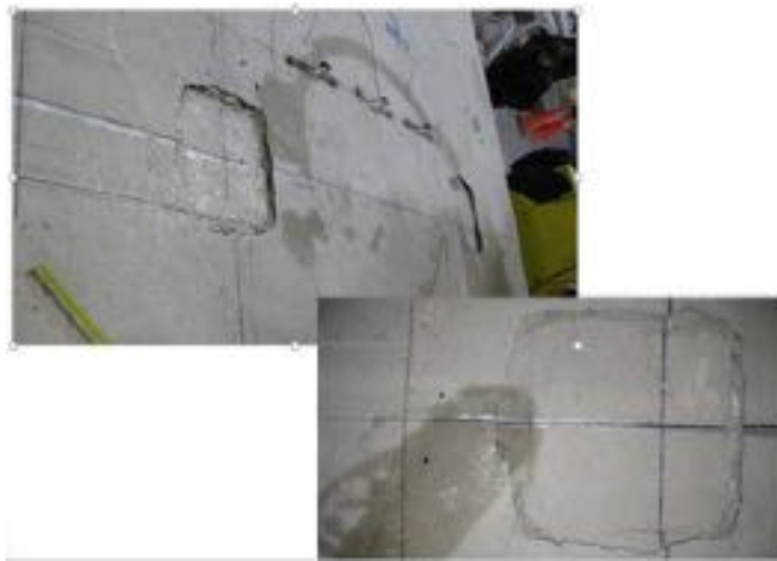
Figure 2-36. Punching shear failure in the Test E-2 of FIU bridge.
