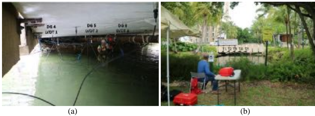
Figure 3-7. Installed instruments. (a) Dial gauges 4 to 6 and LVDTs 1 to 3; (b) Total-Station and targets T1 to T5.
