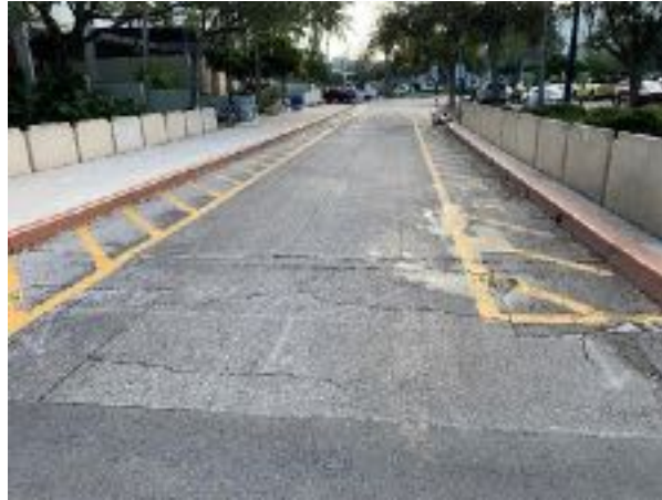
Figure 1-6. Reflective cracking on the deck surface of a precast bridge.
