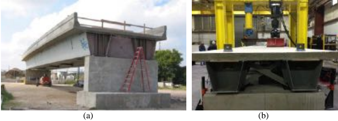
Figure 1-4. Twin steel box girder bridge tests; (a) University of Texas at Austin, (b) Florida International University.
