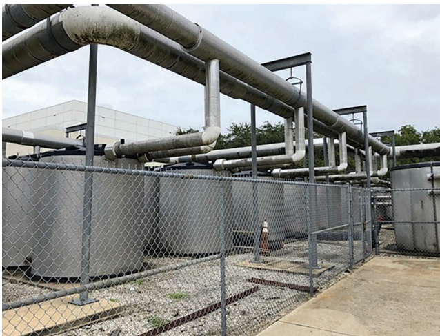
FIGURE 11.2 Ice storage tanks for off-peak load shifting.
