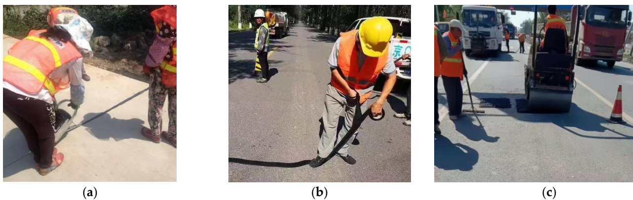
Figure 1. Traditional repair methods of crack and pothole: (a) pouring cracking, (b) sealing cracking, (c) digging-patching of potholes. (@Tai'an City Fang Shuo Engineering Materials Co., Ltd.).
