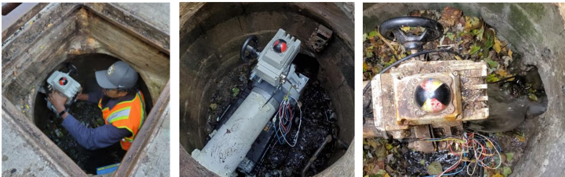
Figure A 4-4. Active control installed at the underdrain of the green alley.
